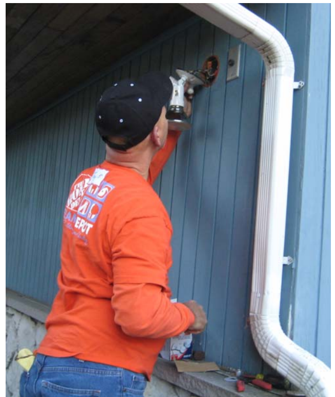
Honeywell volunteers install a new hand rail in Greenlake (left). RTS Board member, Anne Quigg, tours home repairs with veteran homeowner, Earl, in Shoreline (upper right) while a Home Depot volunteer replaces a broken light (lower right).
